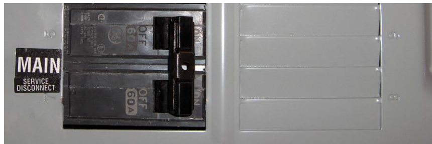
Figure 58 - Breaker box Service Disconnect on left. Photo by N5IUT
